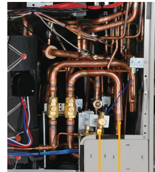
Liquid pipe Gas pipe
